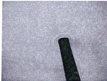
#5 Water Heater Exhaust
